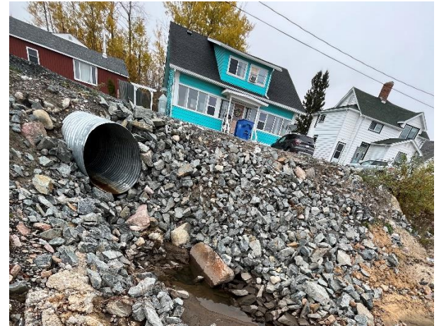
Photo 12: Looking east at Culvert Outfall 01; the outlet was clear and local riprap was observed around it.
