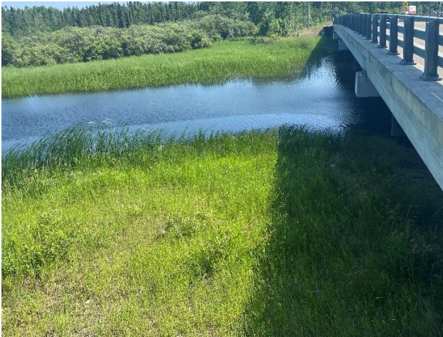
Photo 1: Looking south at the east side of the bridge at Pelican Creek.
