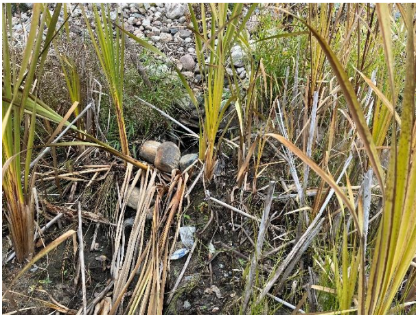
Photo 9: Culvert Outfall 03 along the shoreline west of Pelican Creek; the outlet was dented and silted in.
