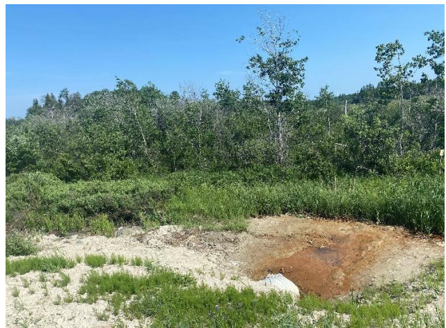
Photo 6: Looking southeast at the culvert outlet south of Ed Ariano By-Pass (Culvert is east of the bridge).
