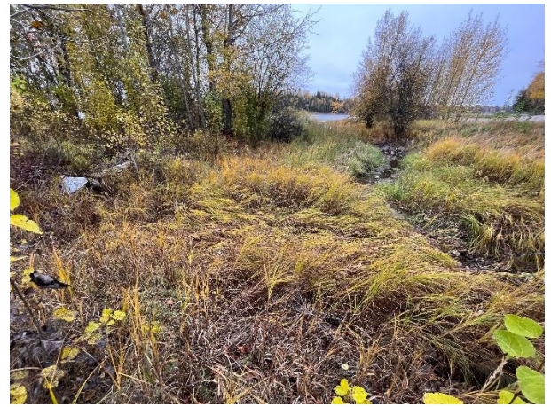
Photo 10: Culvert Outfall 02 across 4 th Ave; the outlet was dented and excessive vegetation was observed.
