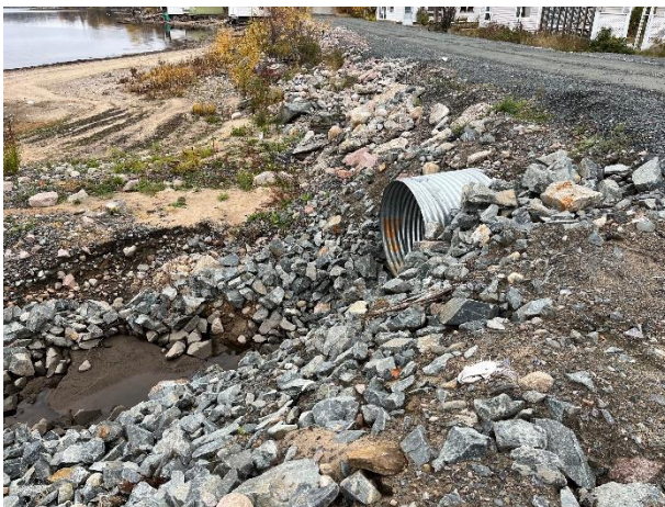
Photo 11: Looking northwest at Culvert Outfall 01 across Lakeshore Dr north of Honey Ln along Sioux Lookout Town Beach.
