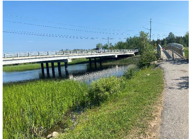
Photo 2: Looking southeast at the west side of the bridge at Pelican Creek.
